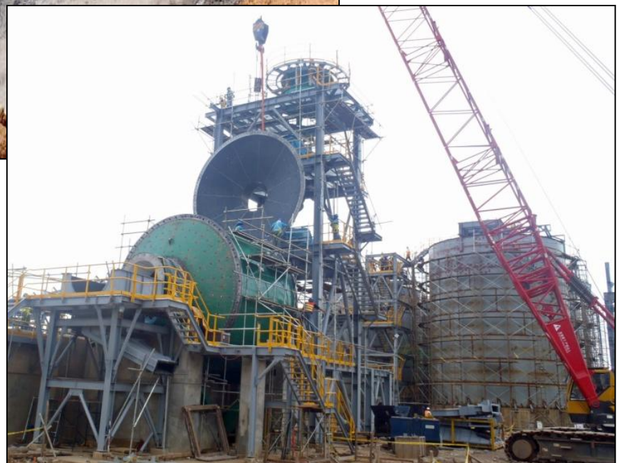
Final steel structural components for cyclone and gravity tower, and installation of SAG mill (Source: RED 5)
